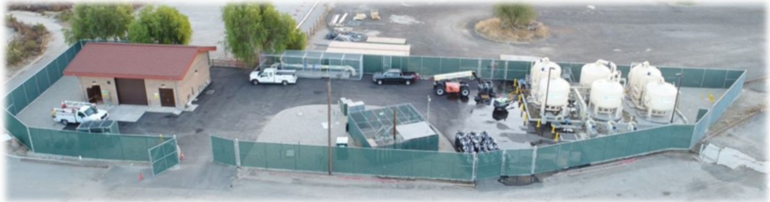
N Wells - Ion-Exchange PFAS Treatment Vessels
