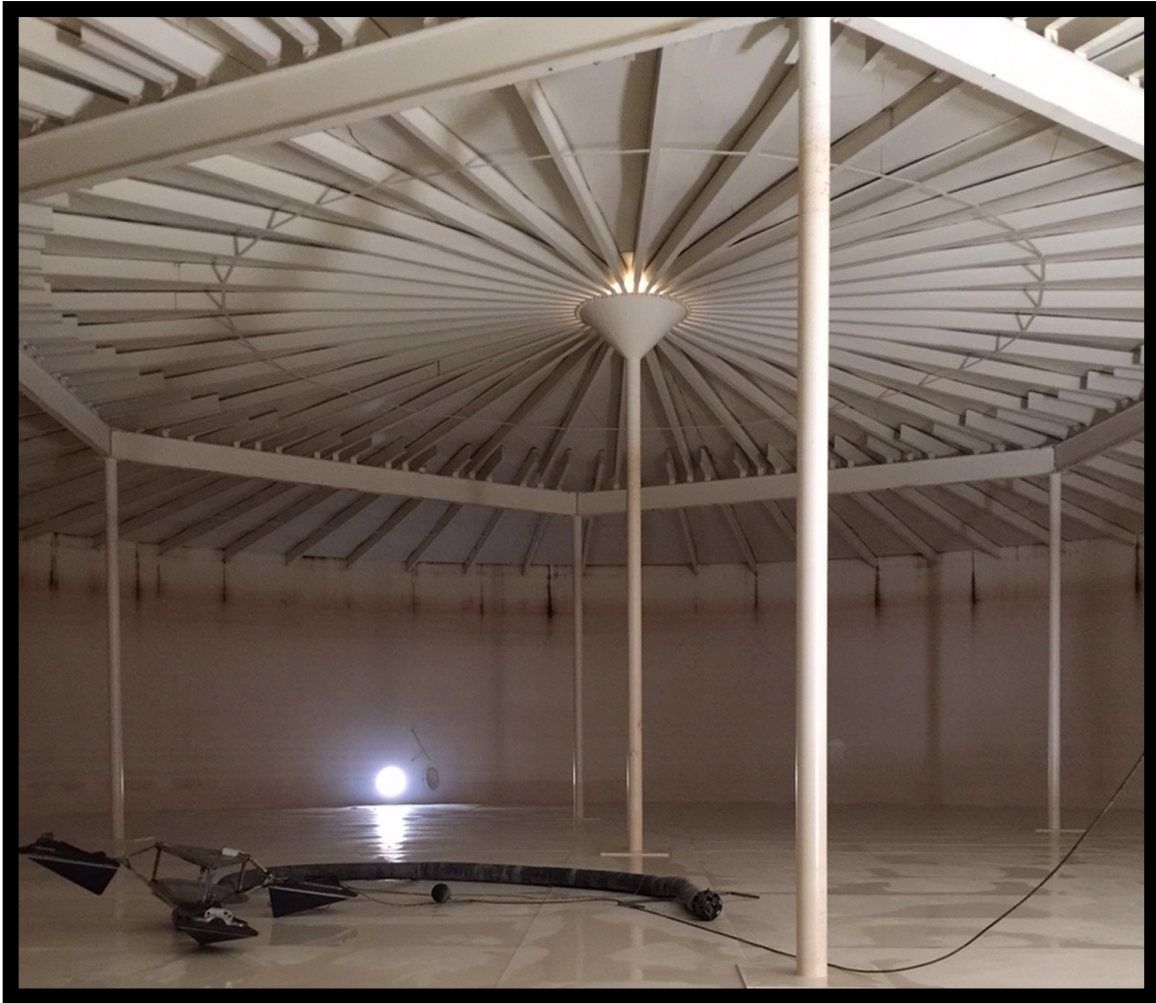
SolarBee mixing unit inside an empty potable water tank (above).
