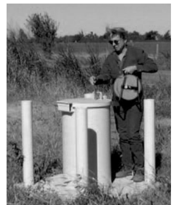
Groundwater Observation Well
