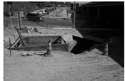
Installation of a conveyance pipeline in the City of Santa Clarita by Castaic Lake Water Agency
